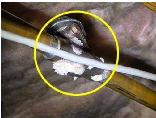
Photo 46-1 THIS IS THE CHECK VALVE ABOVE THE WATER HEATER.
