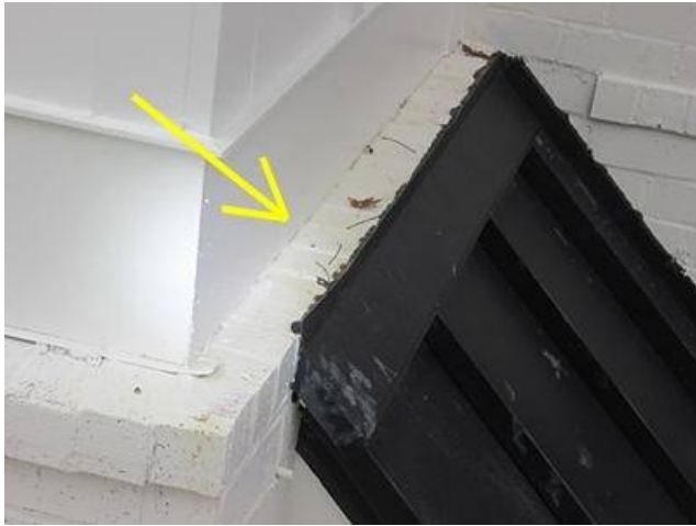
Photo 9-2 LEDGE ABOVE THE BASEMENT ENTRY DOOR.
