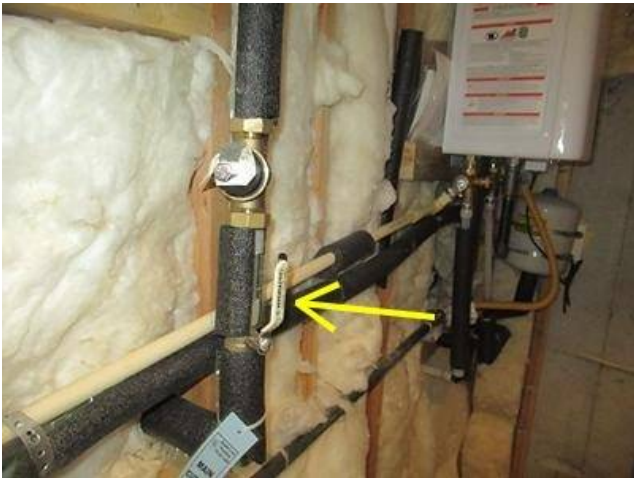
Photo 56-1 BASEMENT UTILITY ROOM IN THE GARAGE.
