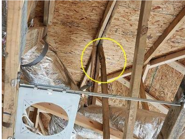
Photo 4-4 LOCATED ABOVE THE MASTER BATHROOM AND MASTER CLOSET AREA.
